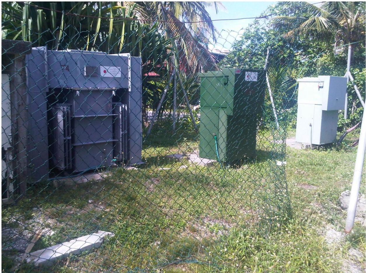
Figure 3 – Typical RMU with switches
