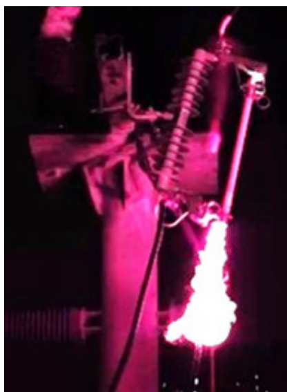
Fig. 1: A night photo of a rewirable DDO fuse in operation
