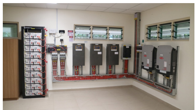
Figure 8 Inverters and Battery System for building
