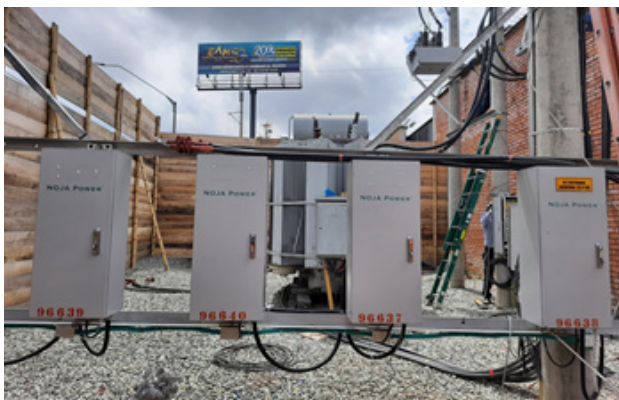
NOJA Power's RC-10 Recloser Controller in use at an EDEQ substation - level I of automation through SGA.
