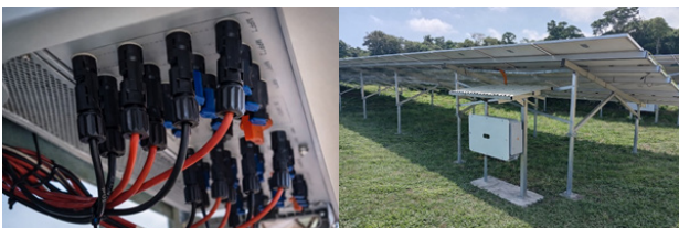
Grid integration included Huawei inverter systems and SCADA monitoring for operational performance tracking.
