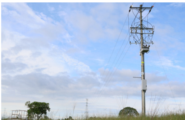
NOJA Power's OSM Recloser and Recloser Controller in a rural site in Quindío, Colombia.
