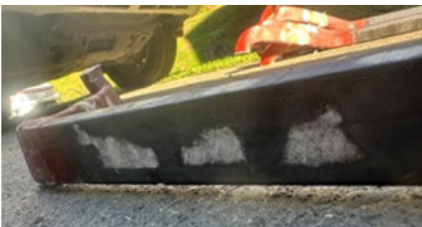
Removed Unit 3 coil showing PD-related damage
