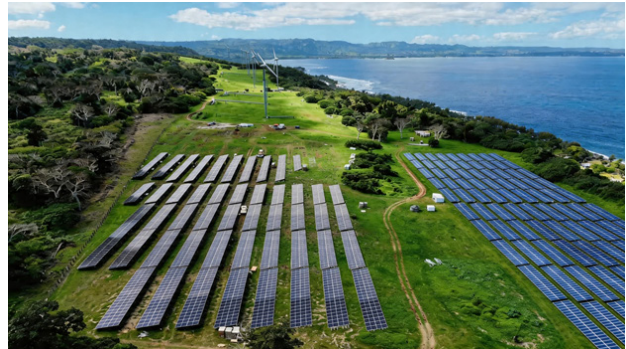
The completed 3 MW Kawene Solar Farm on Efate Island contributes renewable generation capacity to Vanuatu's electricity network.
