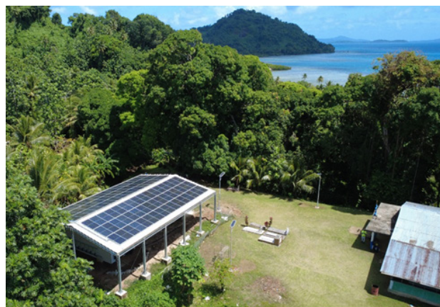
Figure 2. Solar mini-grid in Monowe, Udot, Chuuk
