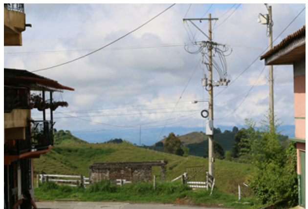
NOJA Power's OSM Recloser and Recloser Controller in a rural site in Quindío, Colombia.
