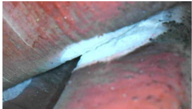
As Found PD-Related damage at coil crossovers
