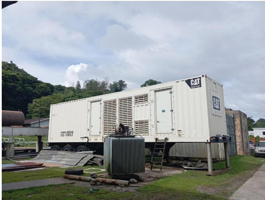
CAT Mobile Genset, 2.0MW 2012
