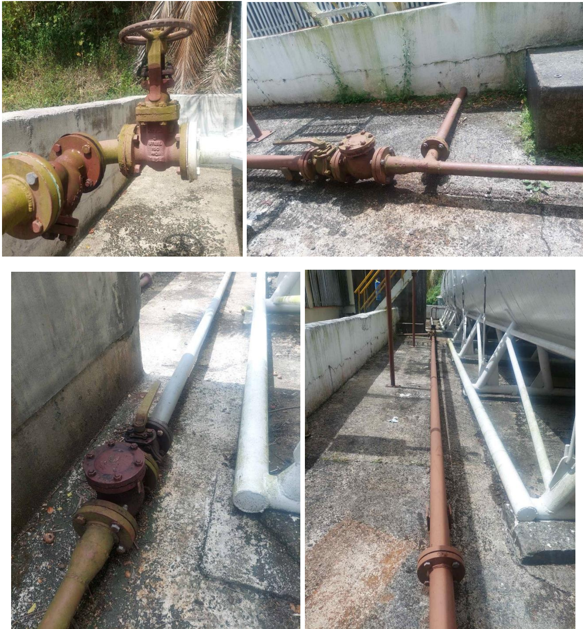
Figure 1: 4" discharge line in tank bund
