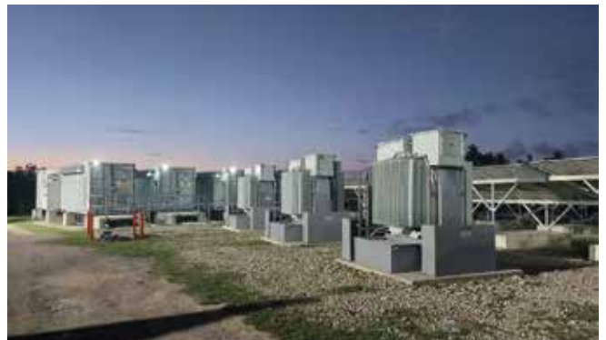
BESS TREP 1 (5 MWh / 10 MW)
