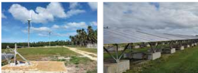
Niuouta wind farm (1.3 MW) and Maama Mai solar facility (1.3 MW) at Popua Power Station
