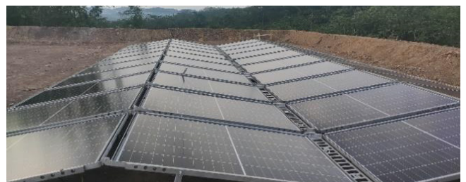
Figure 5 and 6: Deployed "Solar Wings" field from solar containers Mobil-Grid® in Indonesia
