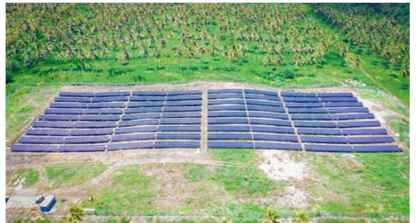
Sunergise Tongatapu 6MW solar farm
