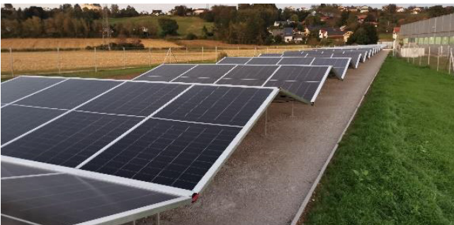
Figure 7 & 8 : 20' container Solarfold® 130kWp – 110 kVA
