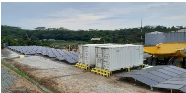
Figure 1: two deployed Mobil-Grid® 72 kWp solar containers in Indonesia
