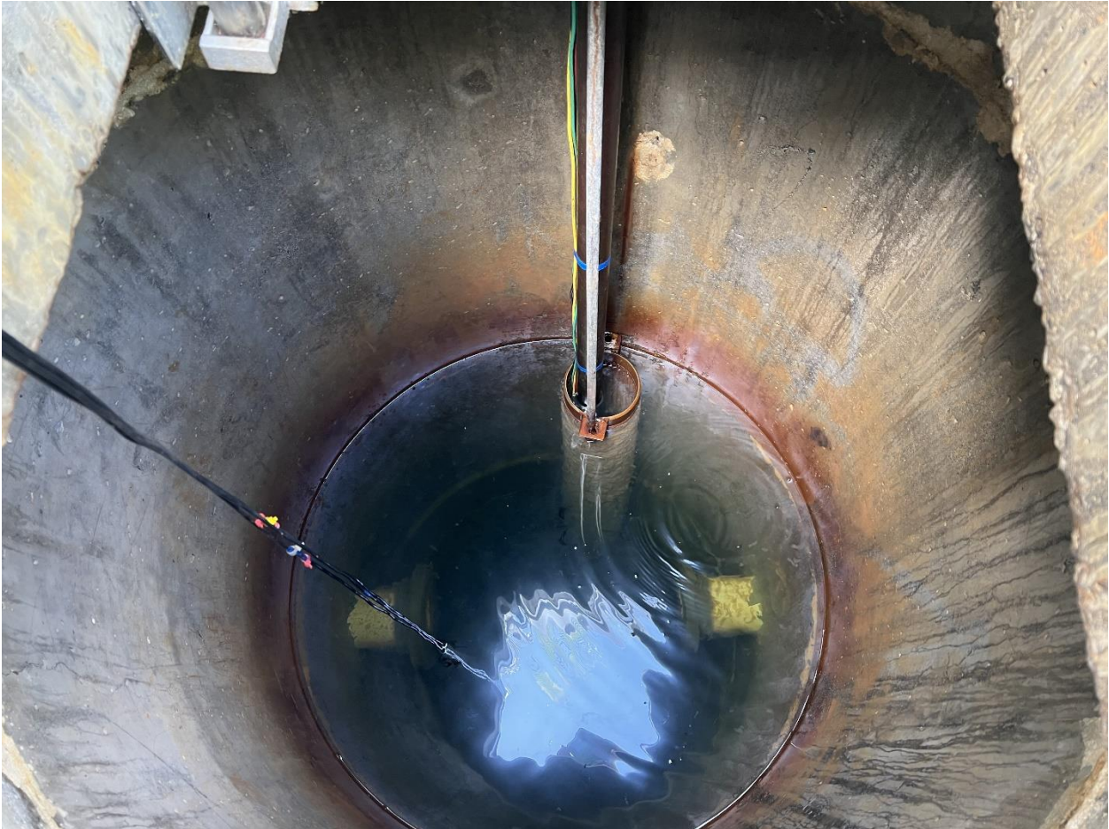
Photo 2: Inside the infiltration gallery on Aunu'u Island.
