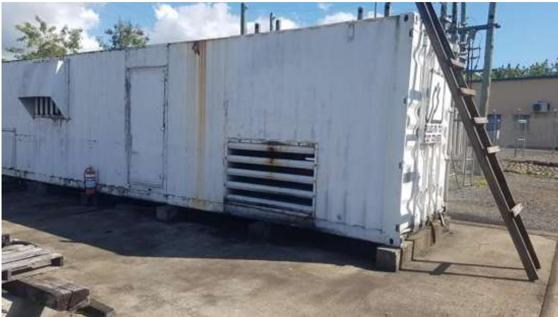
Figure 4: Qeleloa G1. 40 ft containerized generator set
