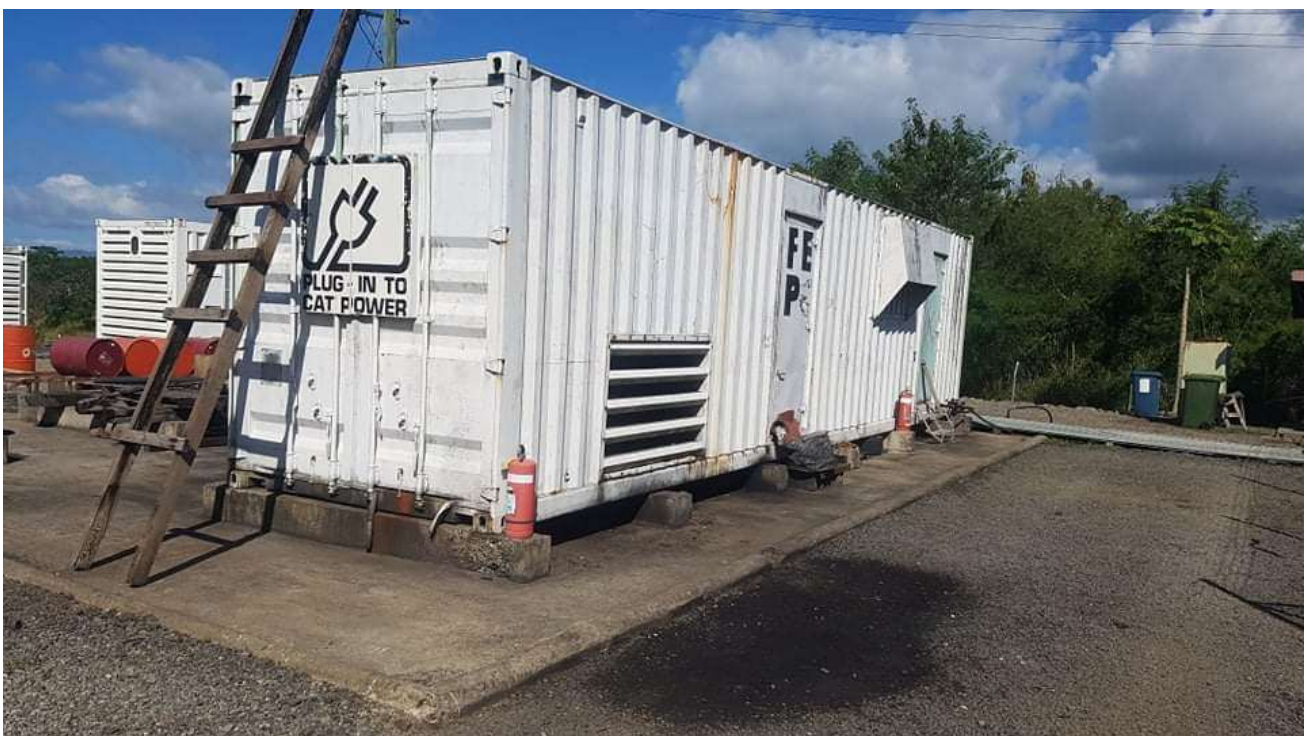
Figure 5: Qeleloa G1.40 ft Containerized generator set
