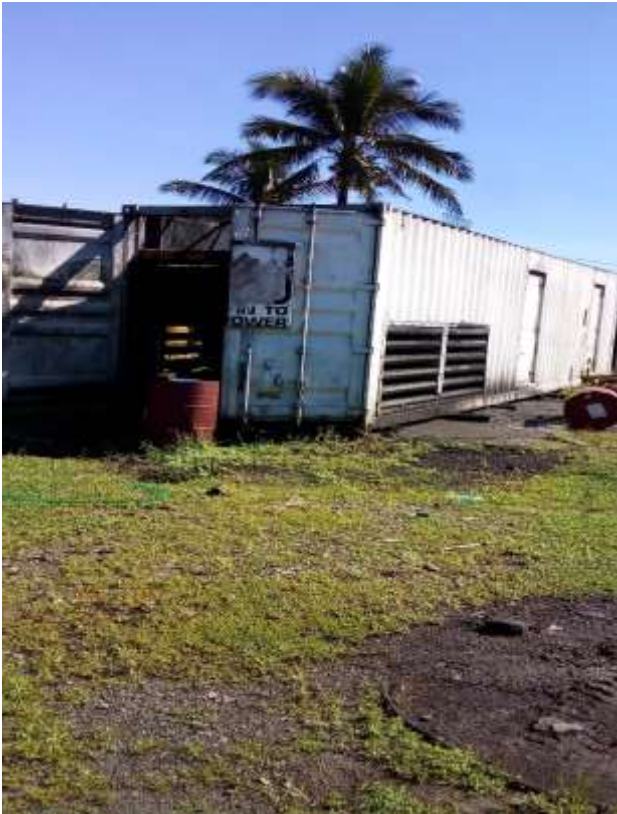
Figure 2: Labasa G10.40 ft Containerized generator set
