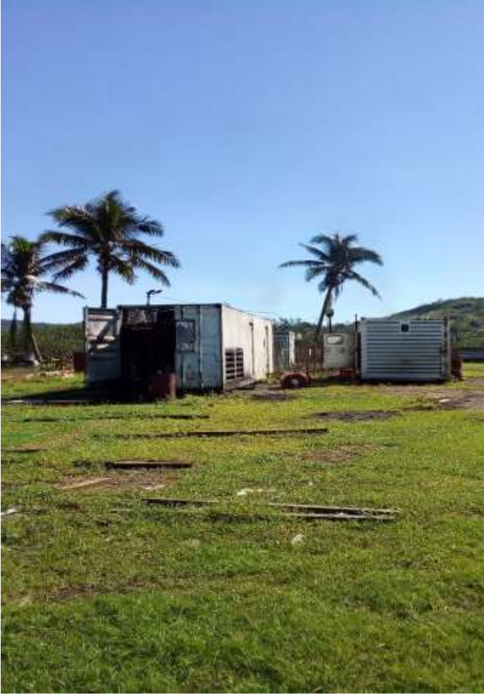
Figure 1: Labasa G10.40 ft Containerized generator set
