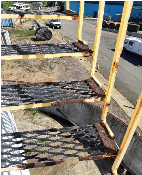
Figure 2: rusted portion of spiral stairway
