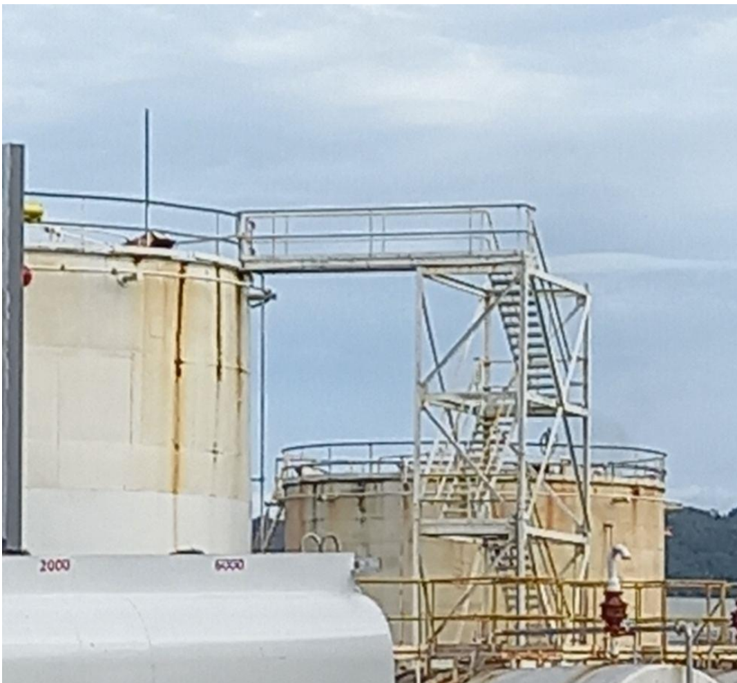
Figure 3: standalone tank access stairway as per the picture below
