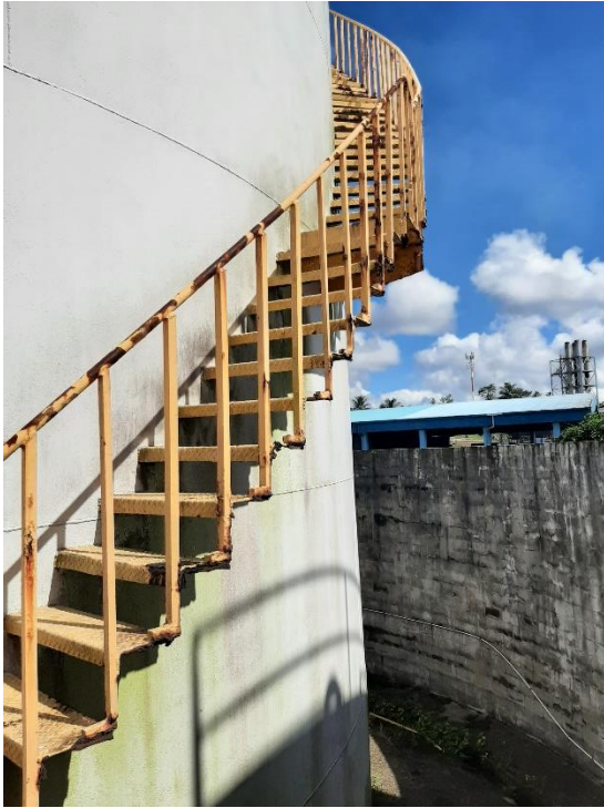
Figure 3: IDO Tank spiral stairway
