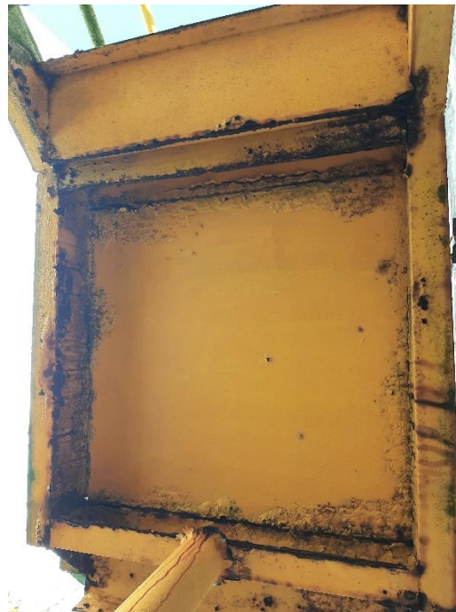
Figure 6: rusted portion underneath Bund wall stairway
