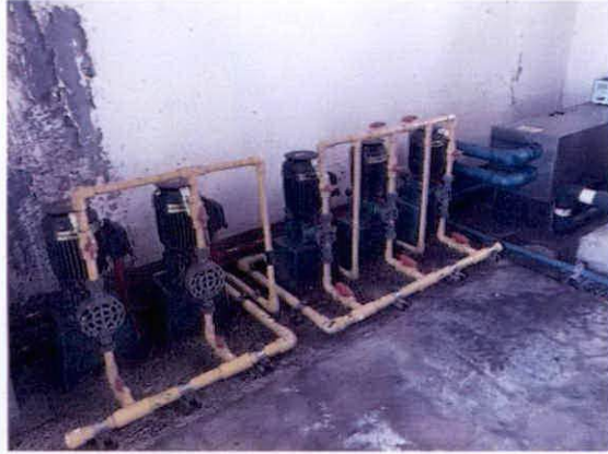
Sludge and equalization tank pumps
