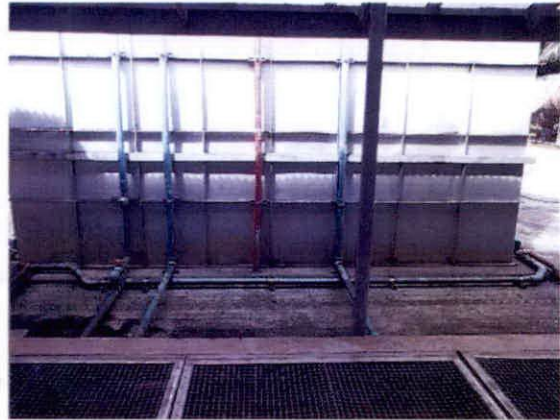
Inlet/Outlet pipes to MBR tank
