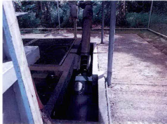
Inlet channel with automatic screen
