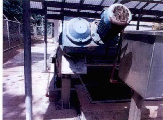
Influent screen pumps
