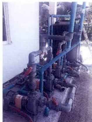
Effluent tank and pumps
