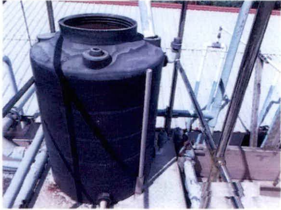
Chemical Dosing Tank
