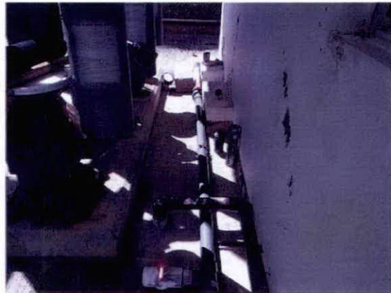
Air blowers and final effluent pipe
