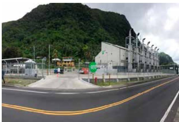
New Satala Power plant
