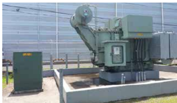
One of two 7.5MVA Tie-Line Transformer at each substation
