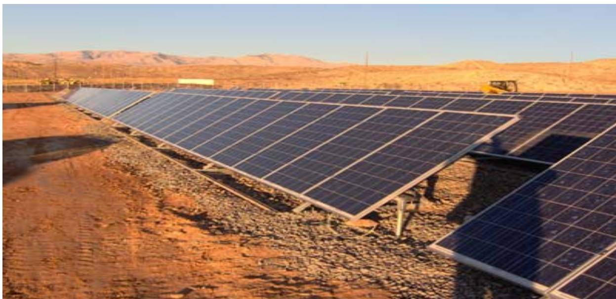
The city of St. George owns a 250-kW solar project called SunSmart PV Facility, above. Photo courtesy of St. George Energy Services Department
